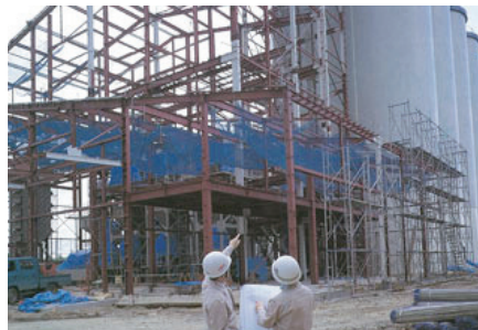
Grain drying and preparation facility
